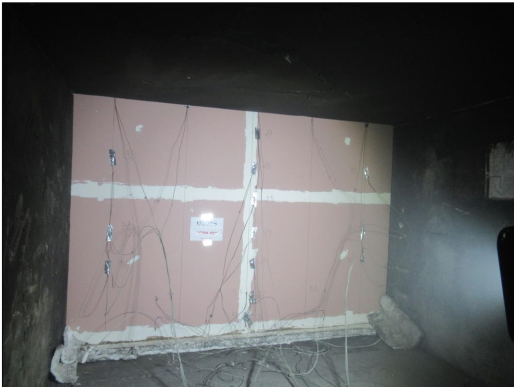
Picture 12: The interior of the base wall in the second floor test room at the beginning of the test.
