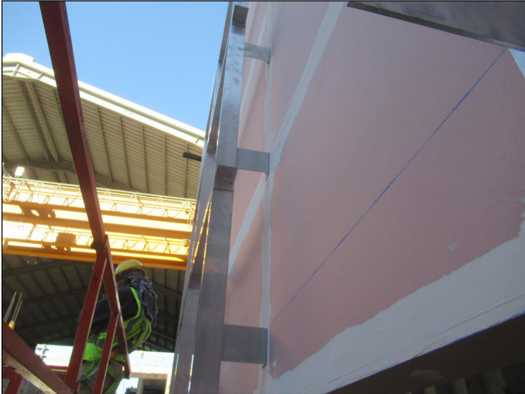
Picture 3: A view of Runners connected to Wall Brackets.
